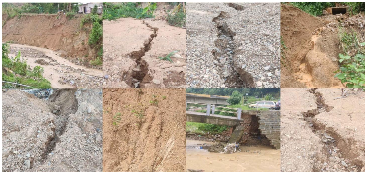
Fig. 4: Photographs of active erosional features in the study area.
